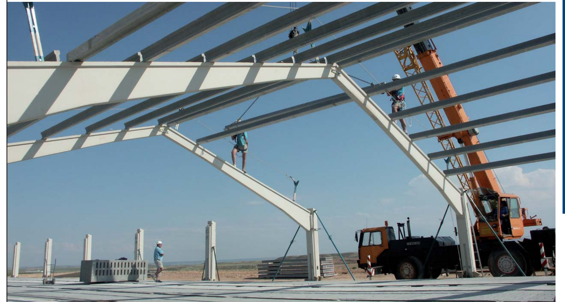
Mounting of cross beams by company fitters using our patented safety system: Ariadna System.
