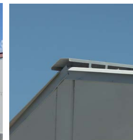
Standard ventilation system
